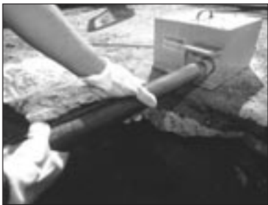
Fig. 5-4. Pipe is typically tapered using one of several power tapering tools available from outside sources.
